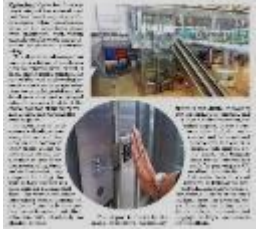
The touch-less elevator at the airport terminal is a testament to the airport's commitment to modern infrastructure and passenger convenience.
